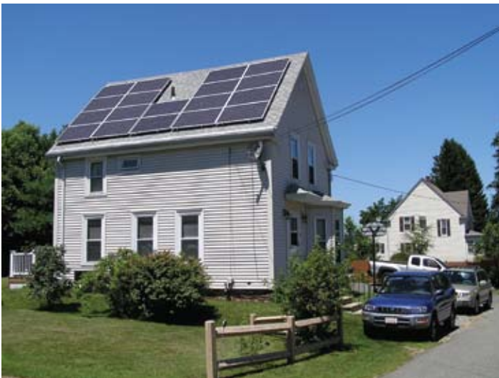
Conti residence's 3.4-kW PV array in Haverhill, MA
