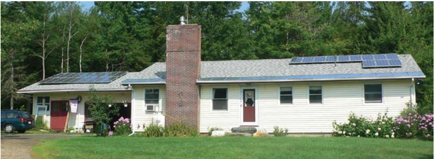
3.45-kW roof-mounted PV array on the Thwing residence in Hawley, MA
