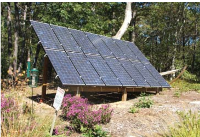
Ground-mounted PV array
